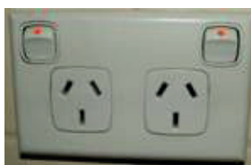
Figure 4: An electrical socket
